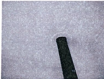
#5 Water Heater Exhaust
